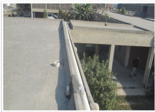
Conveyance pipe around the roof
