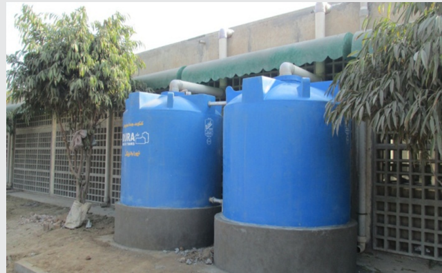
Rain water storage tanks
